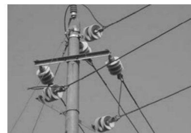
Dead-end for AAC conductor
